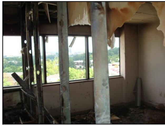
Photo 3. Interior studs of east wall of the fire room that the E1 fire fighter went through to get to the T1 platform at the window. (NIOSH photo)
